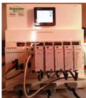
Local control unit
